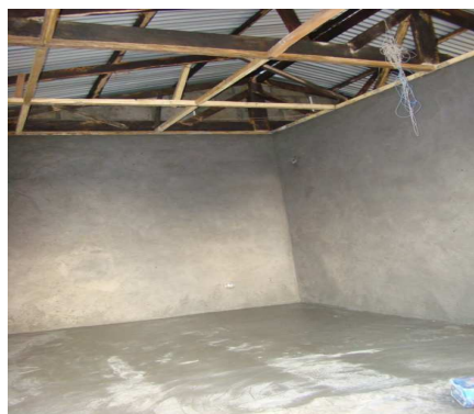
Figure 12 - Inside battery house at Ganta
