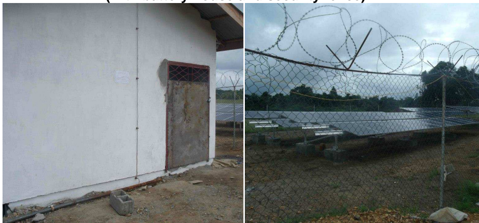
Figure 14 - Harper 20 kW PV system fully installed (with battery house and security fence)
